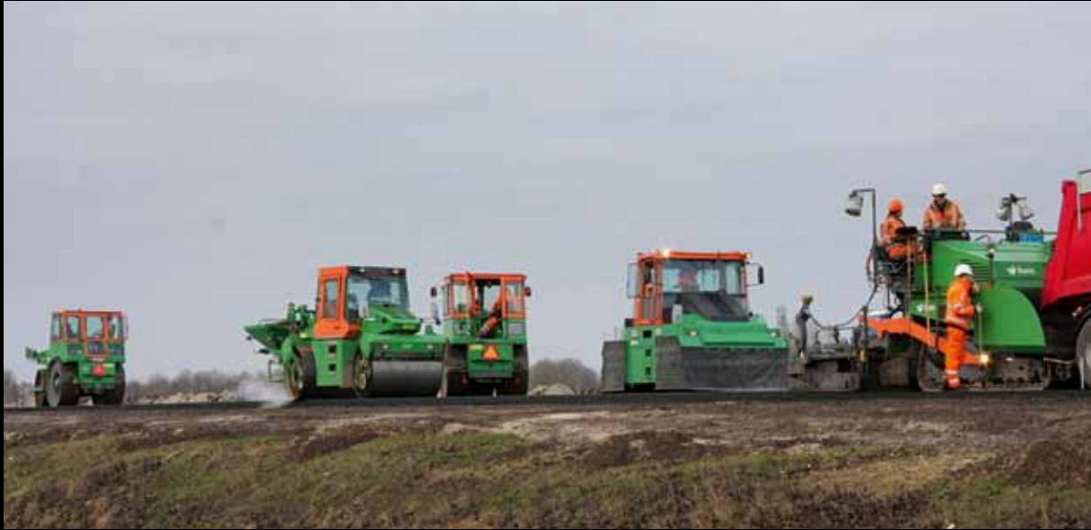
BAM PPP, BAM Civiel, BAM Wegen, BAM Infraconsult. Doubling of the N33 motorway between Assen and Zuidbroek.
