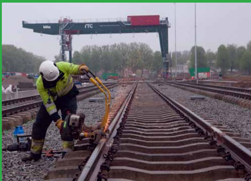
BAM Civiel, BAM Infratechniek, BAM Rail, BAM Wegen, BAM Infraconsult, Betonac. Chemelot rail terminal, Geleen.
