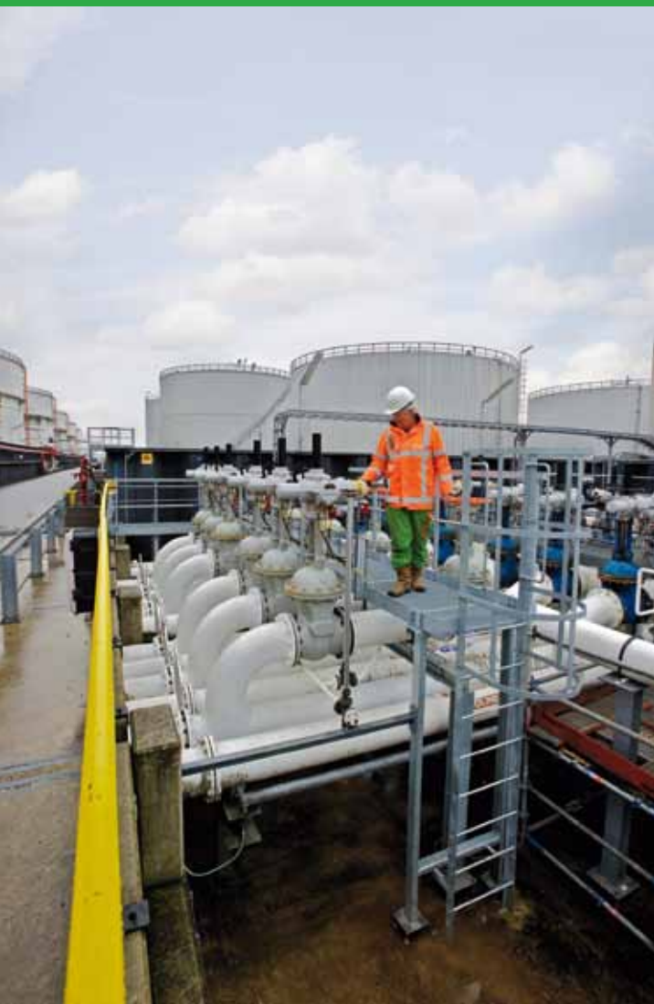
BAM Leidingen & Industrie. New supply pipelines to NuStar Energy L.P. oil supply terminal, Amsterdam.
