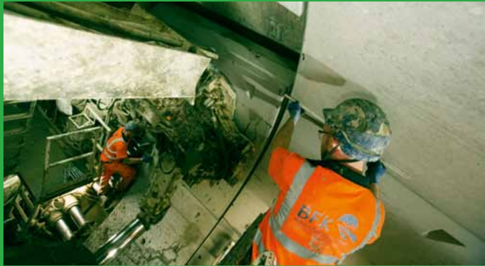
BAM Nuttall, Wayss & Freytag Ingenieurbau (with third parties). Two railway tunnels between the Royal Oak Portal and Farringdon Crossrail stations, London.
